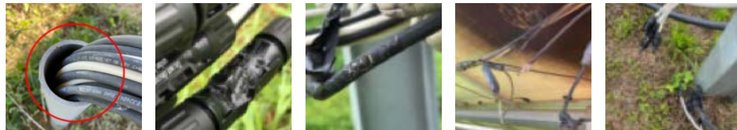
Several issues were found, each contributing to the energy losses the site was experiencing.
